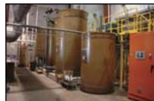
RTF chose its zinc phosphate and black oxide products carefully: effluent in EPA Region 5 is heavily regulated. Above, waste treatment system
