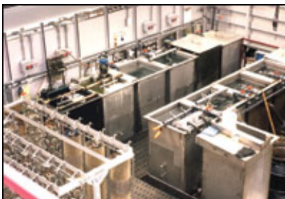
Prototype cleaning line at Electrochemical Finishing (ECF) Grand Rapids, MI, where parts are cleaned prior to plating with electroless nickel.
